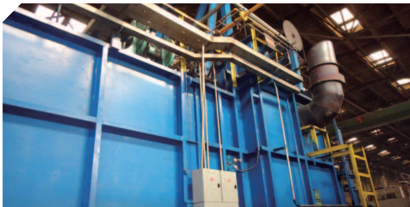
Continuous furnace heating zone energy conversion upgrade project for heat treatment process in CITIC Dicastal
