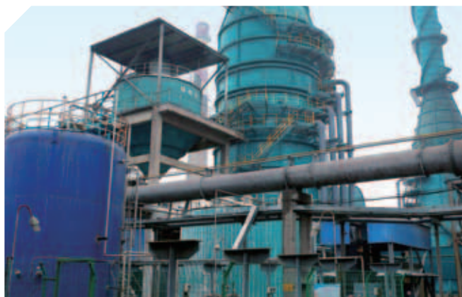
De-sulphuring facilities at Xingcheng Special Steel
