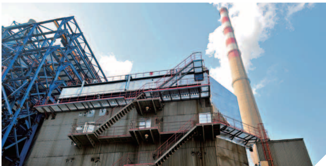
Boiler de-duster upgraded for No. 3 generator (370MW) of Lidian Group
