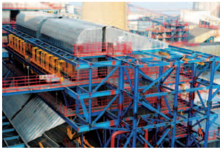
De-sulphuring System in Power Plants
