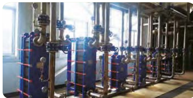
Residual heat recycle and utilization project at CITIC Dicastal
