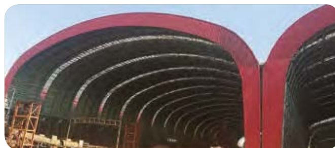
Roofing project of raw material ground by Qingdao Special Steel of CITIC Pacific Special Steel
