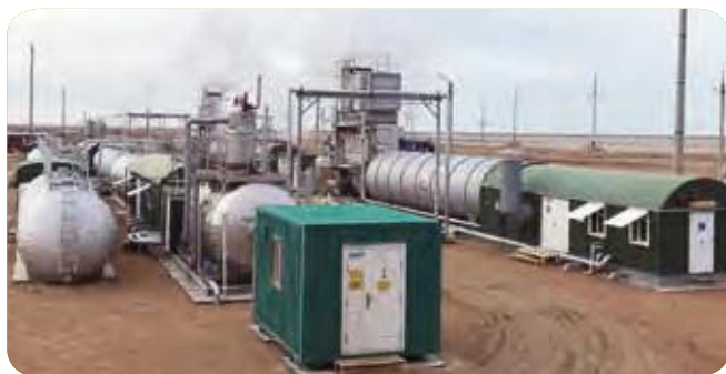
The four energy-saving boilers at Karazhanbas Oilfield
