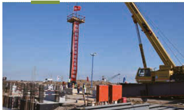
■ CITIC Construction started erecting the steel structure of the combustion engine room at Misan Power Plant in Iraq.
