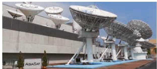
■ Tai Po earth station
