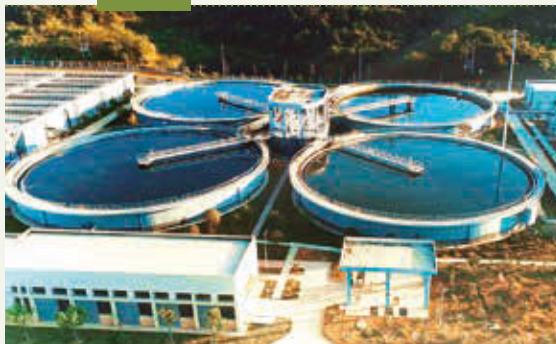
Jiangxia waste water treatment plant
