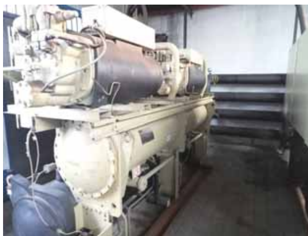
Conversion of residual heat equipment at the east plant area of CITIC Dicastal
