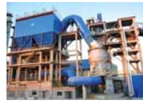
Slag vertical mill (Energy saving and environmental protection)
