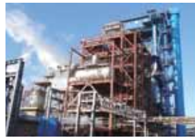
Coke dry quenching waste heat power generation (Energy saving and environmental protection)
