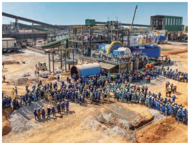
SMPP supply and installation project for the Kipushi zinc mine in the Democratic Republic of the Congo
