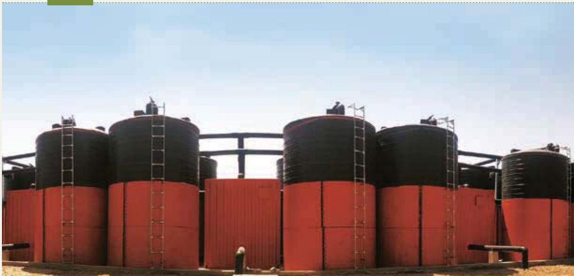
■ Xinji waste water treatment plant of CITIC Envirotech
