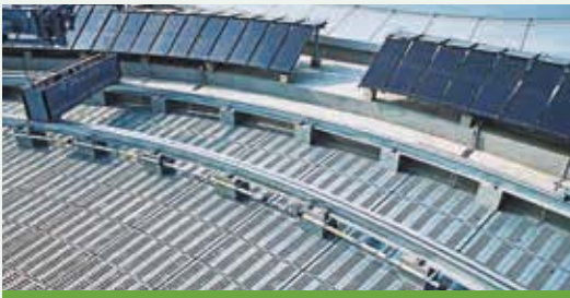
Photovoltaic power generation system at CITIC Tower
