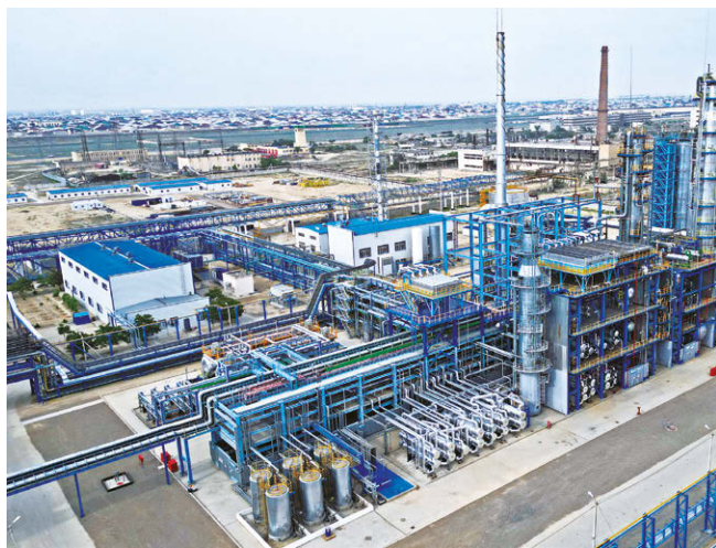
Completion of the reconstruction project for the asphalt plant in Kazakhstan and its commencement of operations
