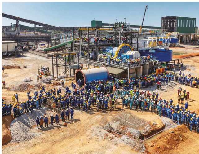
SMPP supply and installation project for the Kipushi zinc mine in the Democratic Republic of the Congo
